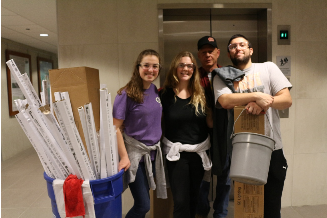
Students and physical plant staff paired up to install nearly 300 tubes for the Main Campus LED Lighting Blitz
