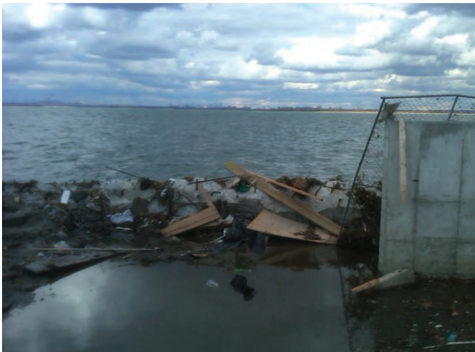
Figure L-07: Thick iron reinforced seawall in the Rockaways broken by force of storm surge (NYSDEC, 2012)
