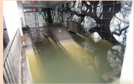
Figure T-03: Escalators under water at the South Ferry subway station. (MTA, 2012)
