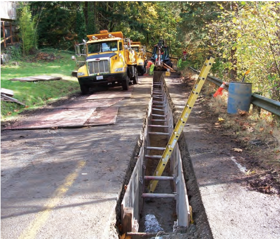
Figure E-07: A Seattle City Light project as an example of selective undergrounding of a power line with frequent outages (City of Seattle, 2012)
