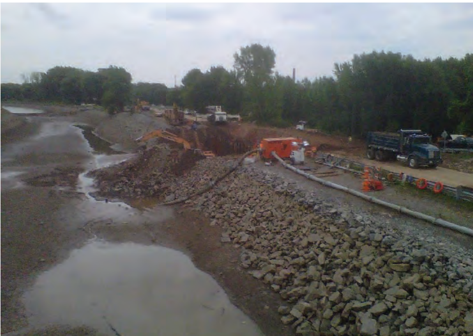
Figure T-20: Emergency repairs at the Erie Canal embankment in Albion, NY. (New York State Canal Corporation, 2012)
