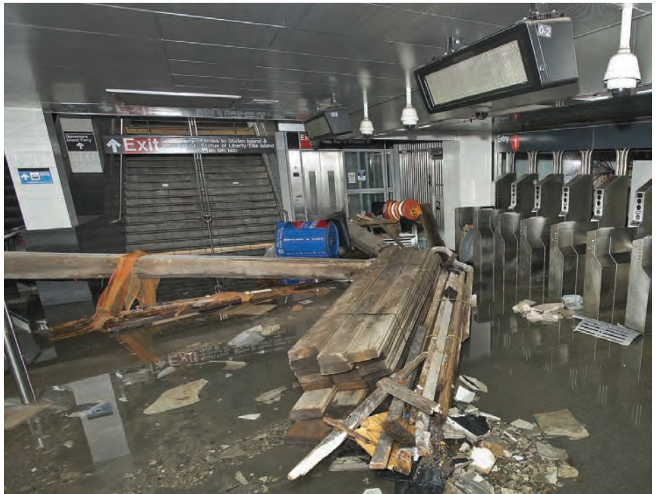
Figure T-12: Damage and debris in the South Ferry subway station following Superstorm Sandy. (MTA, Patrick Cashin, 2012)
