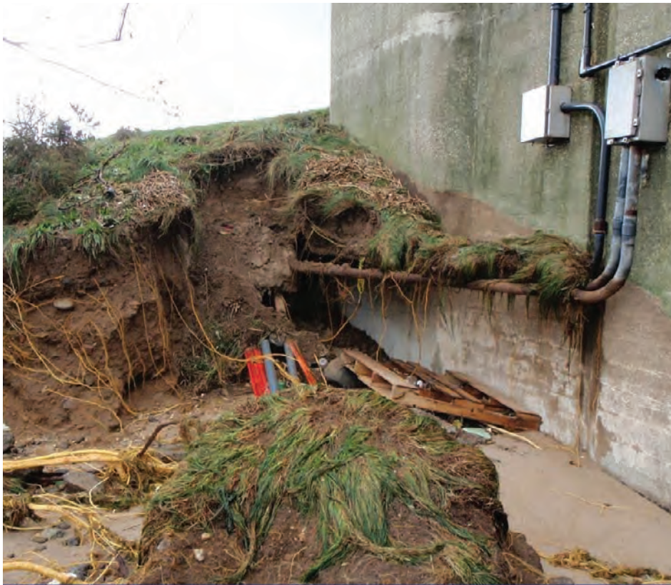
Figure T-17: Bridge scour at the south abutment of the Marine Parkway / Gil Hodges Memorial Bridge in the Rockaways. (MTA, Bridges and Tunnels, Adrian Moshe, 2012)
