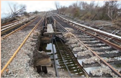
Figure T-01: Damage on the New York City Subway Rockaway Line (A train). (MTA New York City Transit, Leonard Wiggins, 2012)
