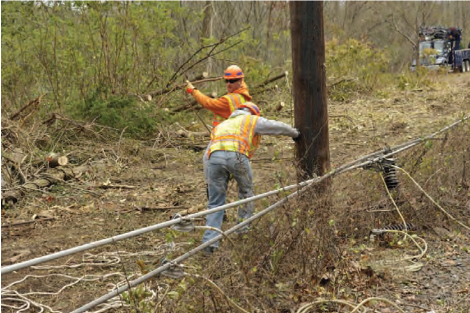
Figure E-06: A hard-to-reach distribution circuit that could be a candidate for selective undergrounding (NYPA, 2012)
