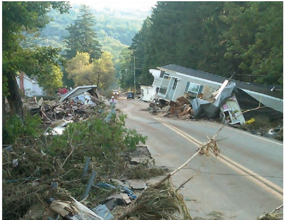
Figure L-22: Destruction and damage from Irene and Lee (NYSDEC, 2011)
