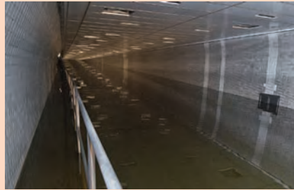
Figure T-02: Superstorm Sandy flood waters run to the ceiling of the Hugh L. Carey Tunnel. (MTA, Patrick Cashin, 2012)
