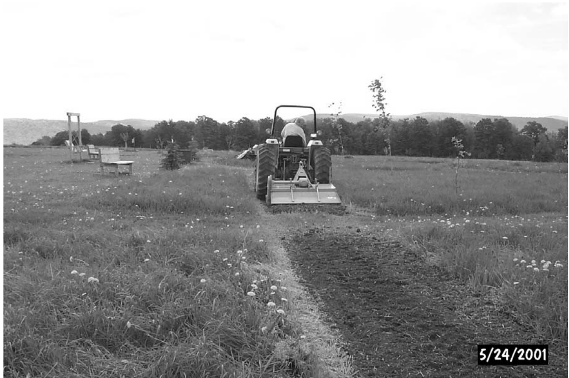
Figure 4. Site preparation at the site of the new living willow snowfence in South Cortland, NY.
